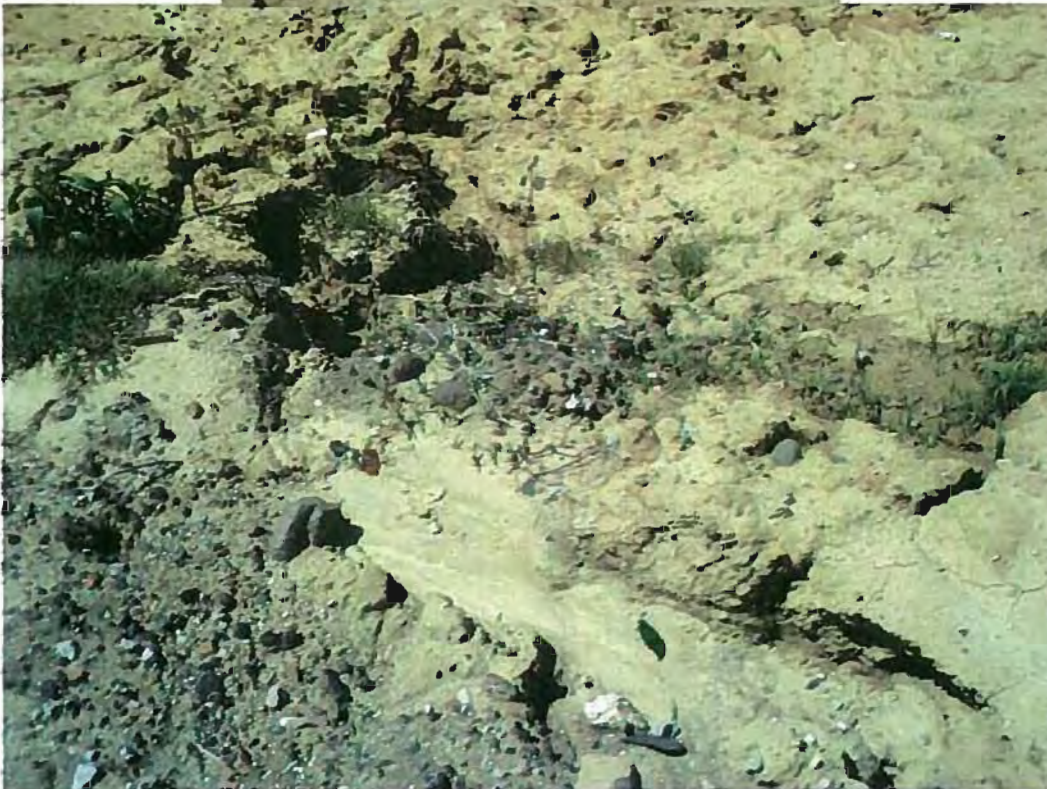
Date: 4/18/2012 Time: 12:52 P.M. Direction: southwest Photo by: S. Williams Exposure #: 018 Comments: erosion gully that continues in photo 019
