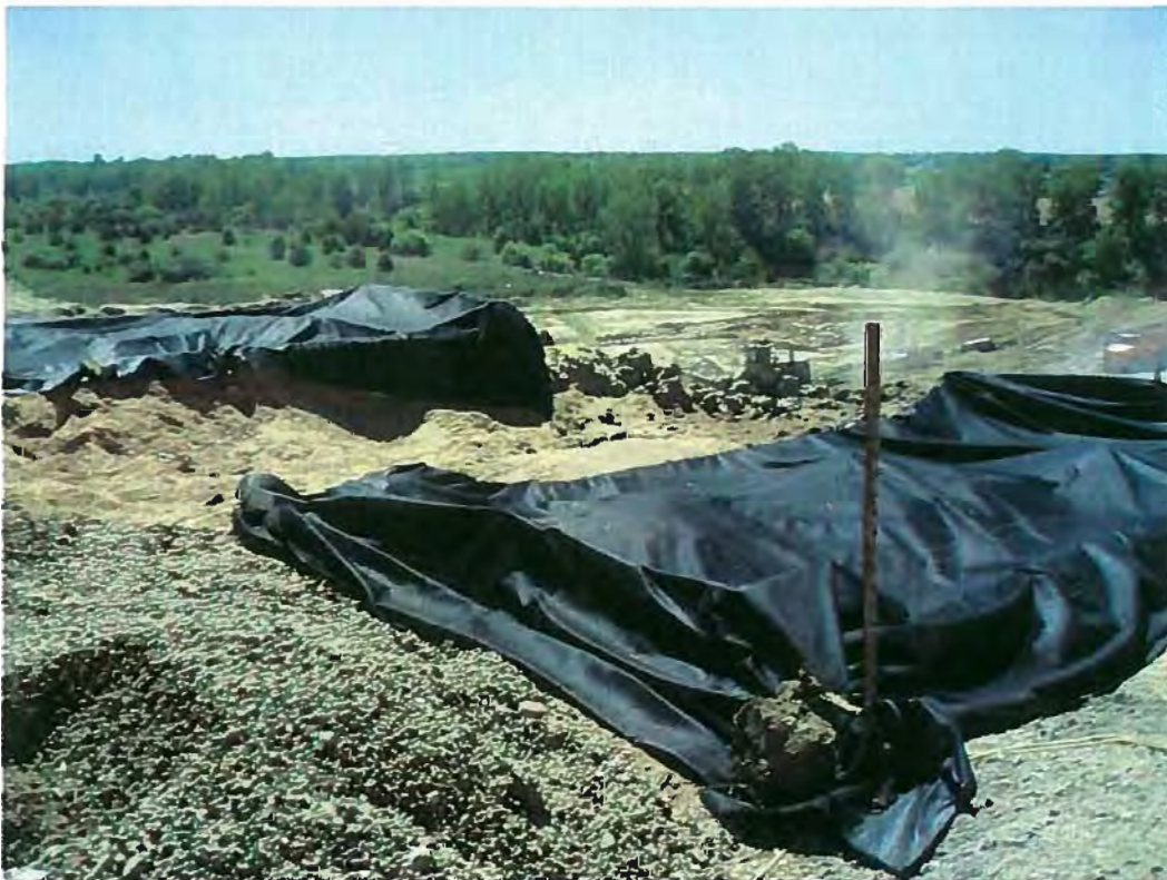
Date: 4/18/2012 Time: 1:39 P.M. Direction: southwest Photo by: S. Williams Exposure #: 022 Comments: new covers on solidification containers
