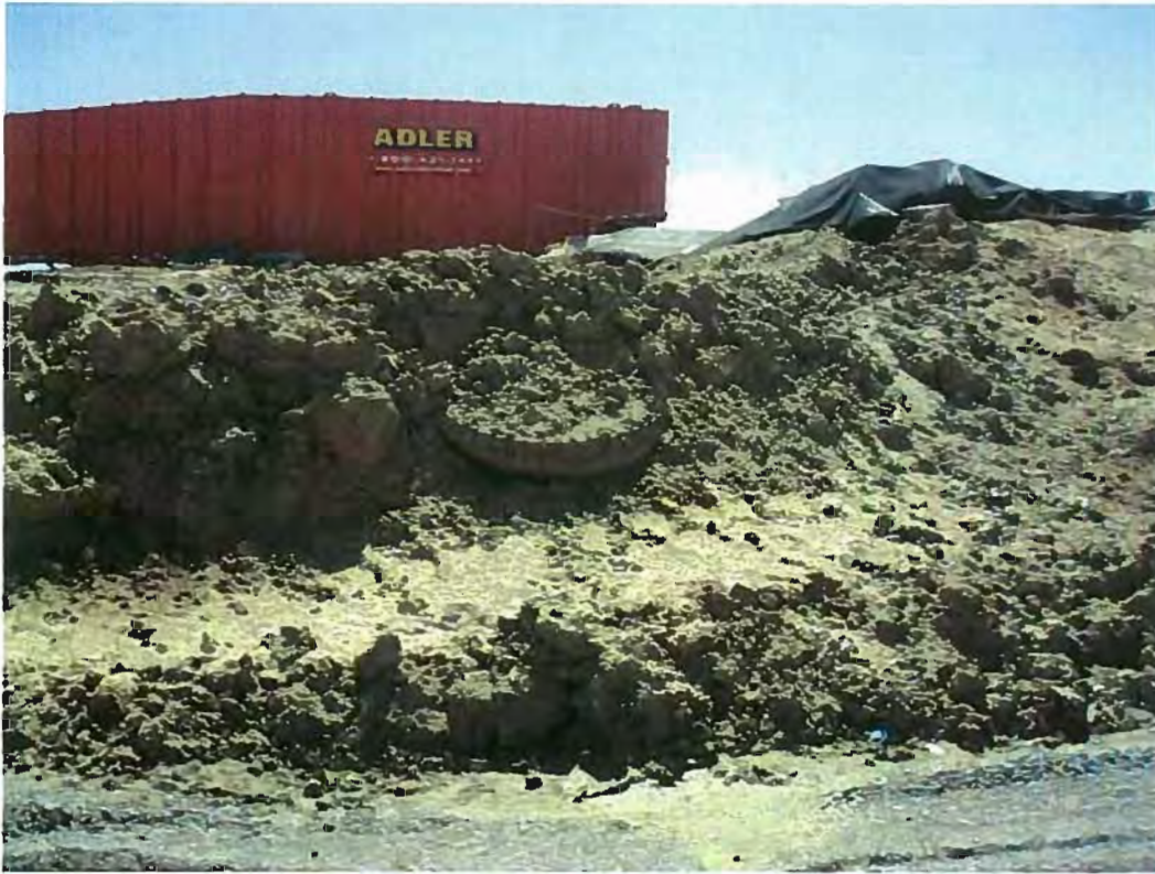
Date: 4/18/2012 Time: 1:41 P.M. Direction: south Photo by: S. Williams Exposure #: 023 Comments: tire protruding from embankment
