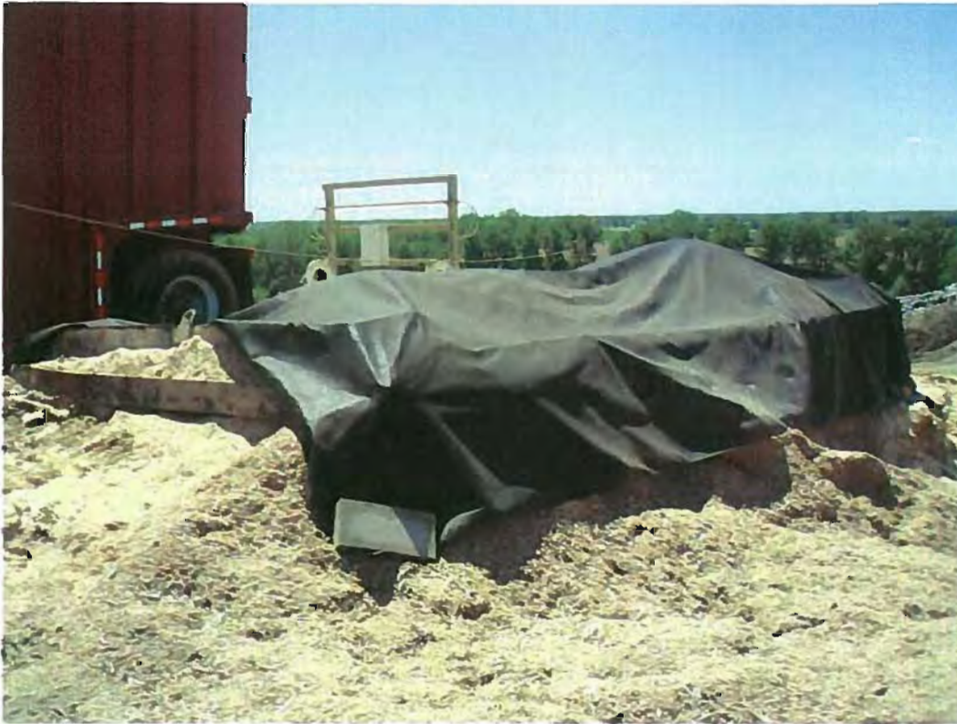
Date: 4/18/2012 Time: 1:38 P.M. Direction: southwest Photo by: S. Williams Exposure #: 021 Comments: new cover placed over some of the waste in the solidification container
