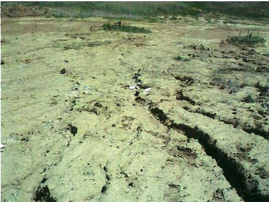
Date: 4/18/2012 Time: 12:06 P.M. Direction: northeast Photo by: S. Williams Exposure #: 012 Comments: erosion gullies
