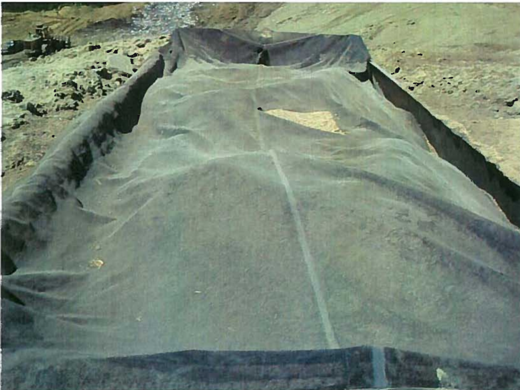
Date: 4/18/2012 Time: 11:08 A.M. Direction: west Photo by: S. Williams Exposure #: 008 Comments: torn & unsecured tarp on solidification container
