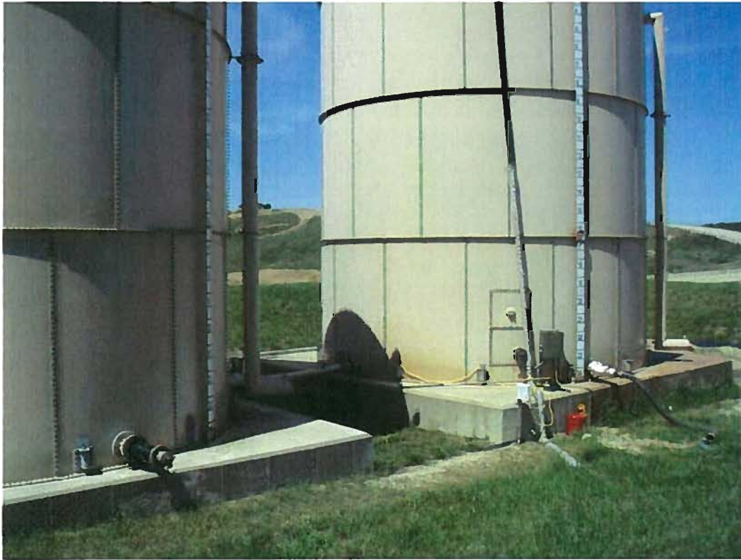
Date: 4/18/2012 Time: 12:28 P.M. Direction: northwest Photo by: S. Williams Exposure #: 015 Comments: gauge on left tank is broken
